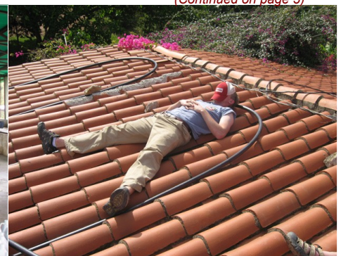
Working hard to install the region's first solar hot water heating system
